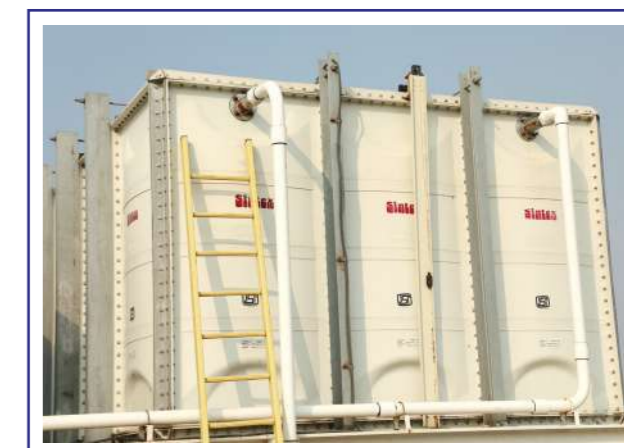
84,000 Litres of tank installed in Leela Business Park, Mumbai
