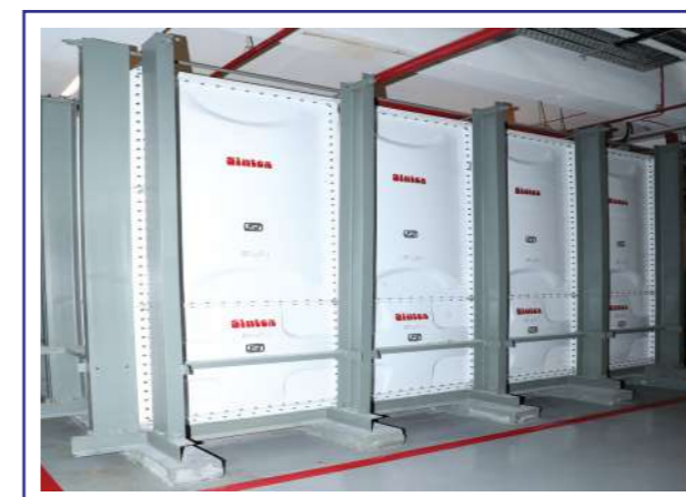
48,000 Litres SMC Panel Tank - Moxy Hotel, Bengaluru
